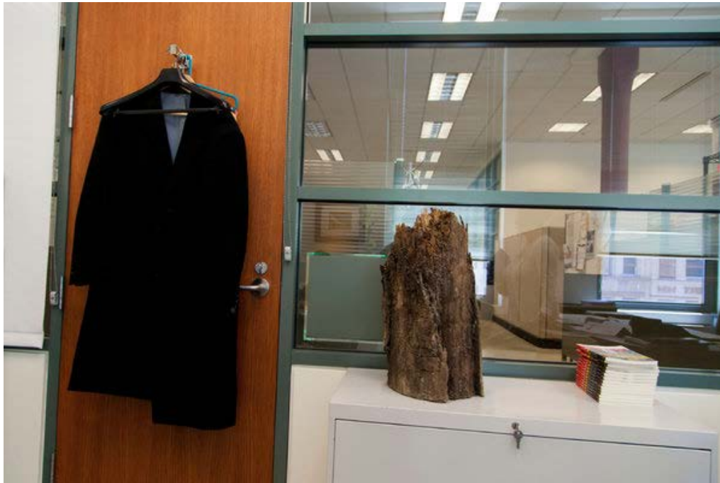
A rotted beam that was removed from the Milwaukee Repertory Theater's substructure and displayed in the office of its managing director, Chad Bauman.
