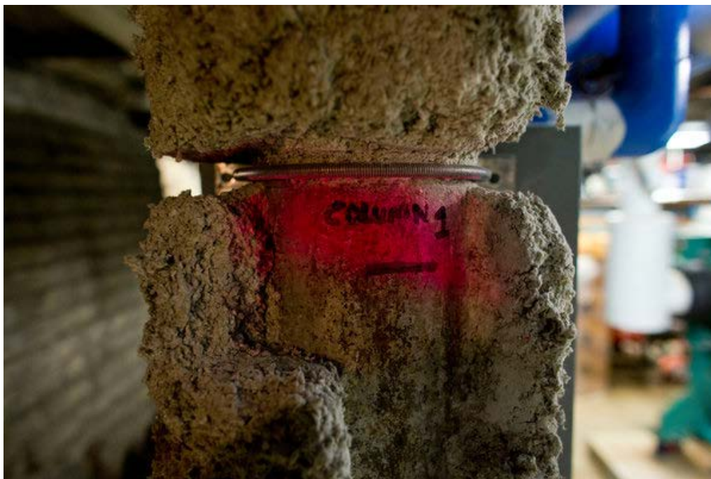
A beam that is part of original foundation is tagged to monitor the rate of sinking. Darren Hauck for The New York Times
