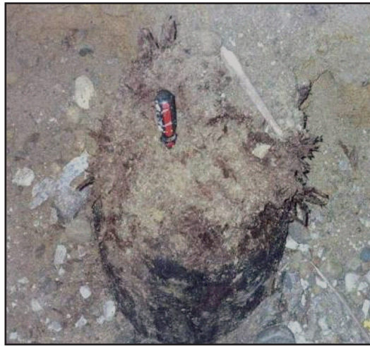
Figure 3: This interior pile, once the column footing was removed, showed no resistance to probing. Groundwater receded a long time ago.
