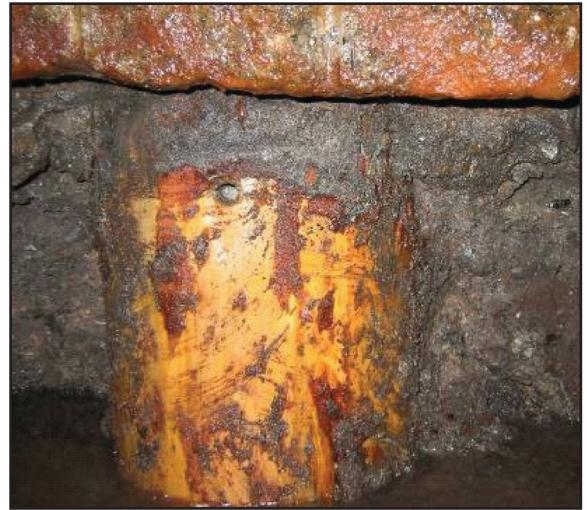
Figure 5: Exposed piles appear to be in good condition. Piles are thought to have continually been in a submerged condition – no damage is expected.
