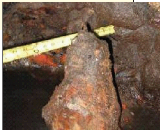
Figure 1: Pile deterioration is so severe that contact with the underside of the pile cap is lost. Note the pencil-top shape indicating attack direction (outside-in).
