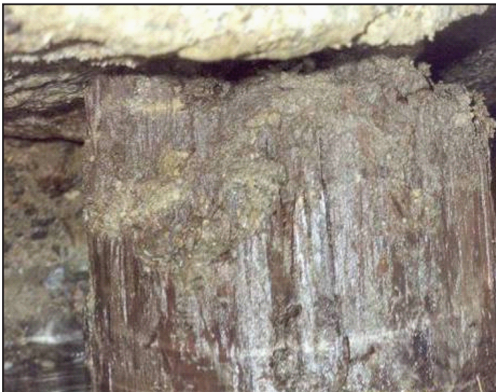
Figure 6: Pile appears in good condition, but later analysis found the pile to be significantly deteriorated. Groundwater is drawn down by pumping.
