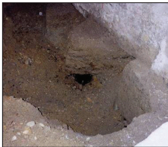
Figure 4: Excavation revealed decayed piles. Groundwater was not encountered and the soil is dry.
